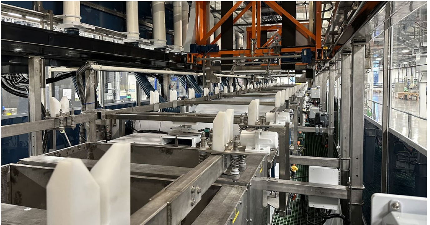
Internal view of IPS automated ENIG line.
