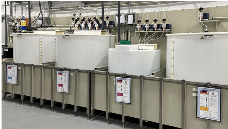
Centralized dosing stations.
