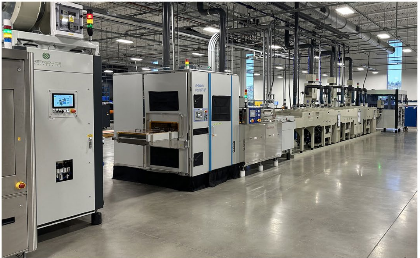
Right to left: GSE double loader, followed by Chemcut preclean line, electrostatic cleaner and preheat oven, cut-sheet laminator, GSE UV-protected lift-up gate, GSE FIFO/FILO-capable buffer with cooling, and partial view of Mylar peeler.
