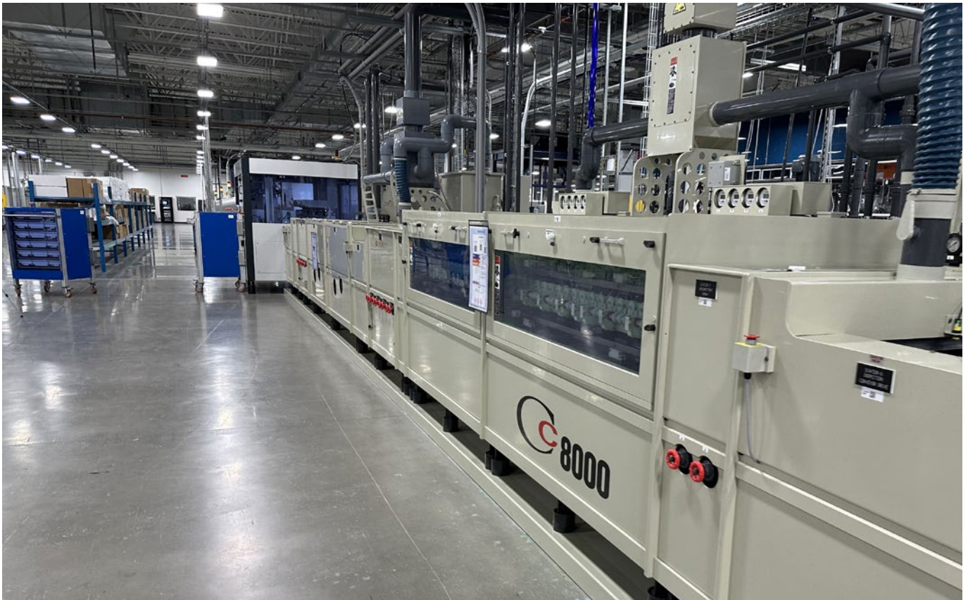
Chemcut CC8000 inner layer develop-etch-strip (DES) system using cupric chloride etchant. The two large portions of the line shown are the etching chambers.
