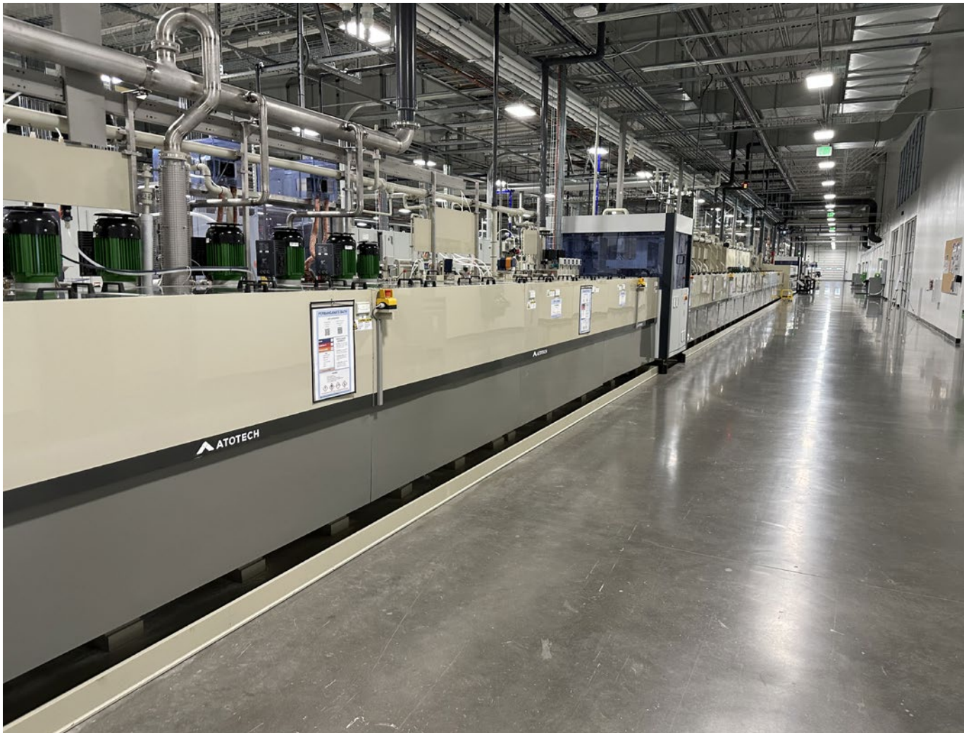
Atotech's 300-foot long horizontal plating line at SEL's Idaho facility.
